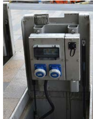
↑ Inground power supply
